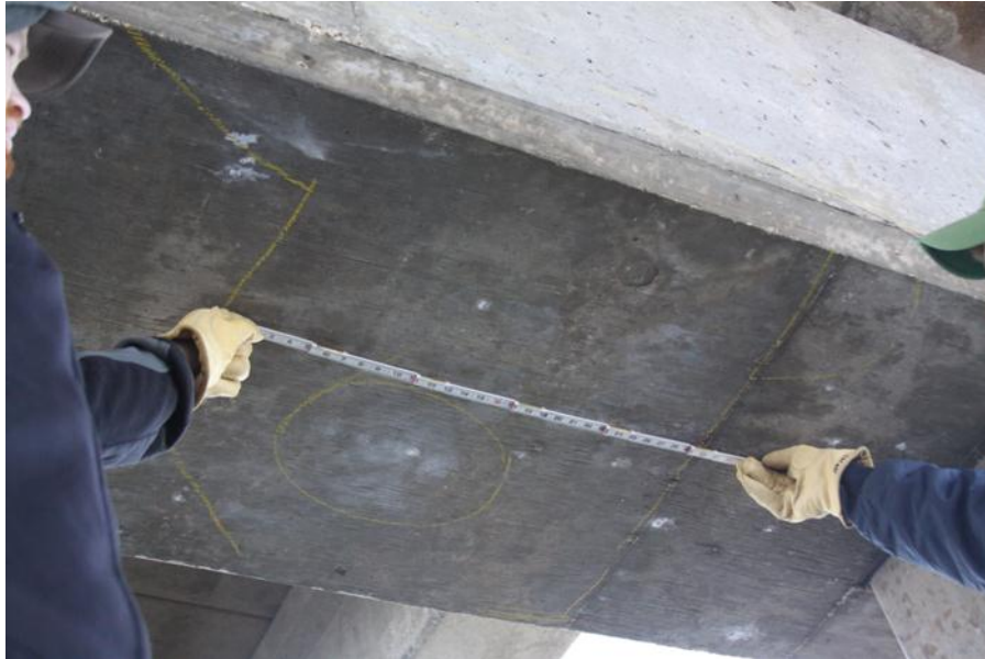
Delamination measurement Digital Image
