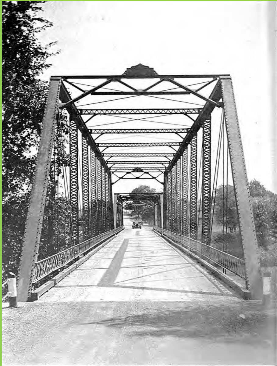
LaBarge Bridge over the Thornapple River. Tightening, strengthening, painting and a new asphalt plank floor brought this bridge up to standard specifications. The work was done this summer, the bridge being closed to traffic only three weeks.
