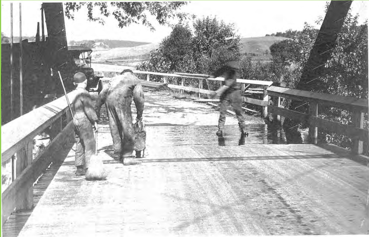
Knapp Bridge—placing seal coat of tar on new floor to waterproof the surface.
