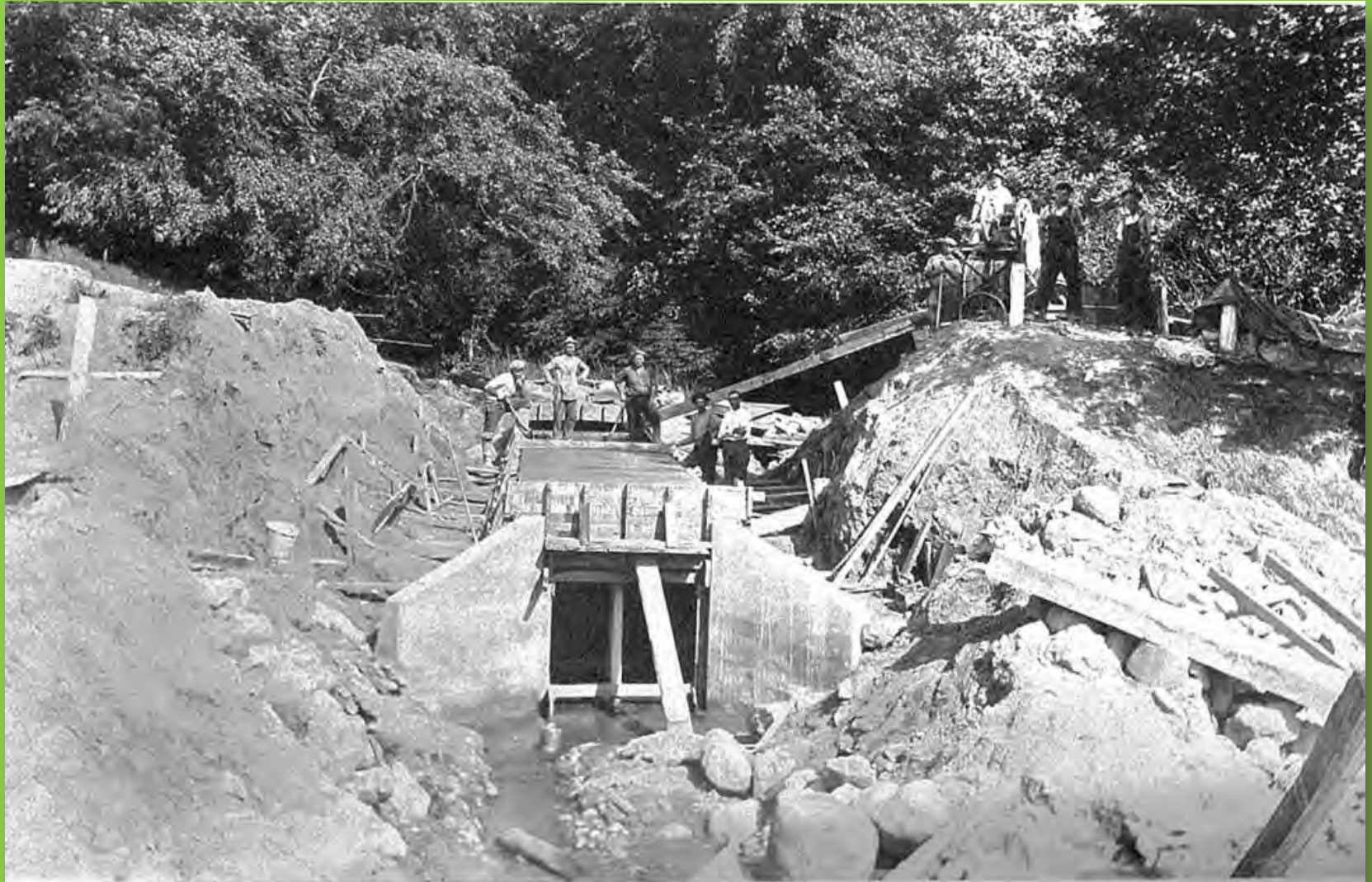
A typical reinforced concrete box culvert under construction on M-13 south of Grand Rapids.
