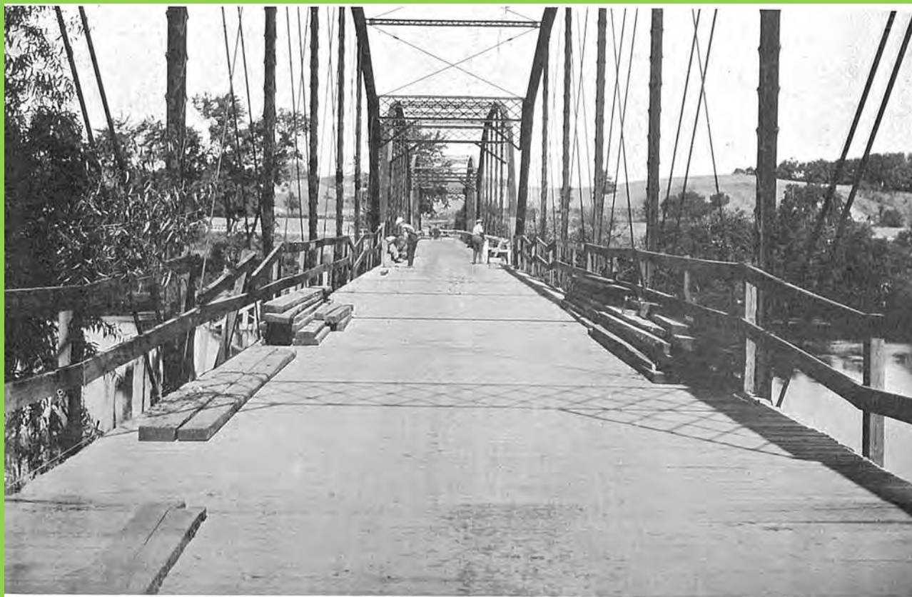
Placing new floor and guard rail on the Knapp Bridge over Grand River. Traffic was not interrupted while this work was being done.
