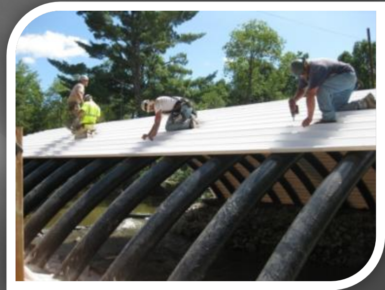
Arches and decking are the only formwork needed to stabilize the structure
