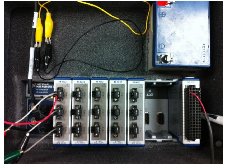
Data acquisition system used to record the signals from sensors
