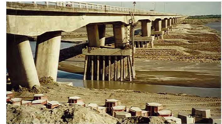
Extreme scour. (Source: Melville and Coleman)
