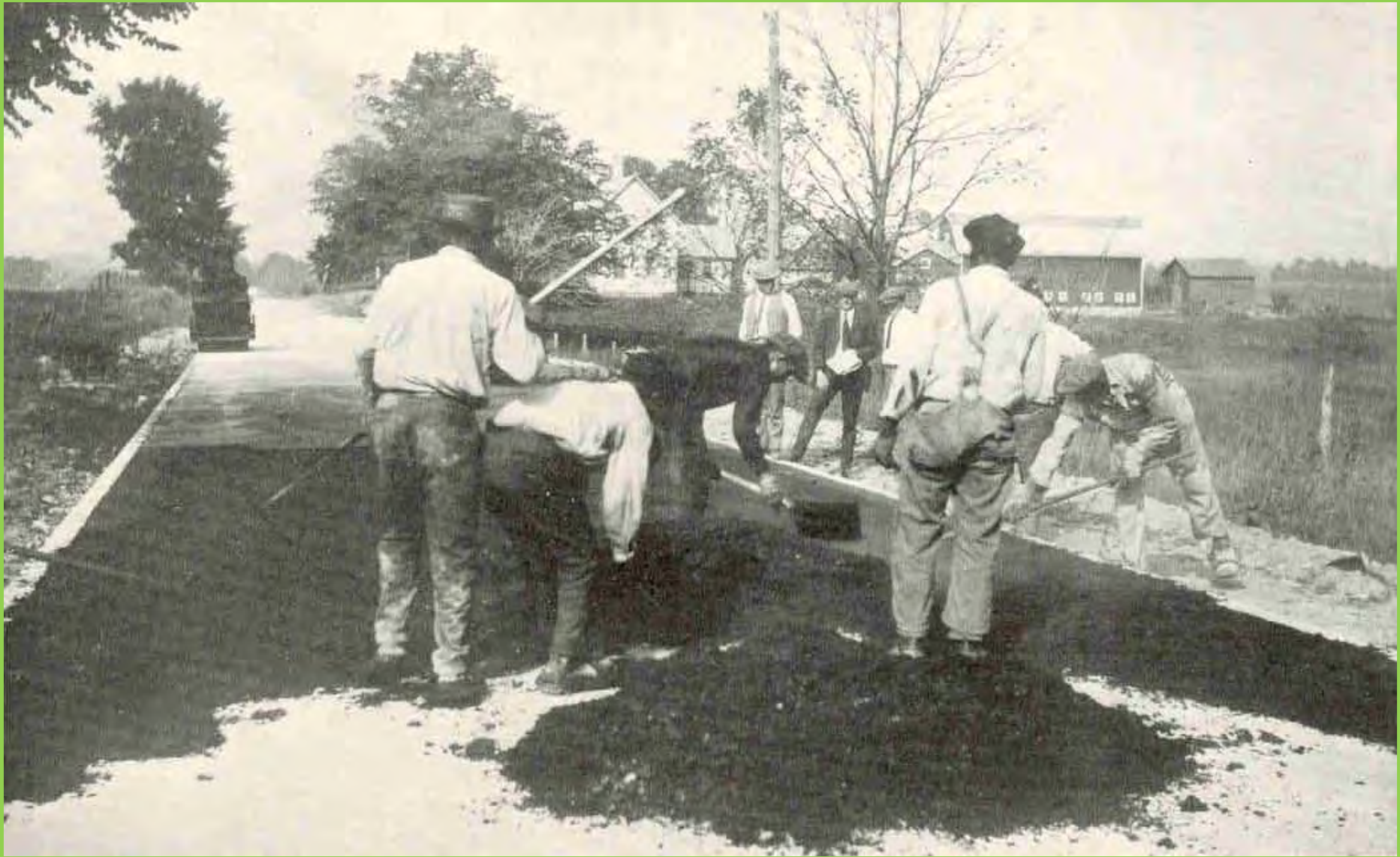
It's an "Armstrong paver" – asphalt mixed on site in a concrete style batch mixer
