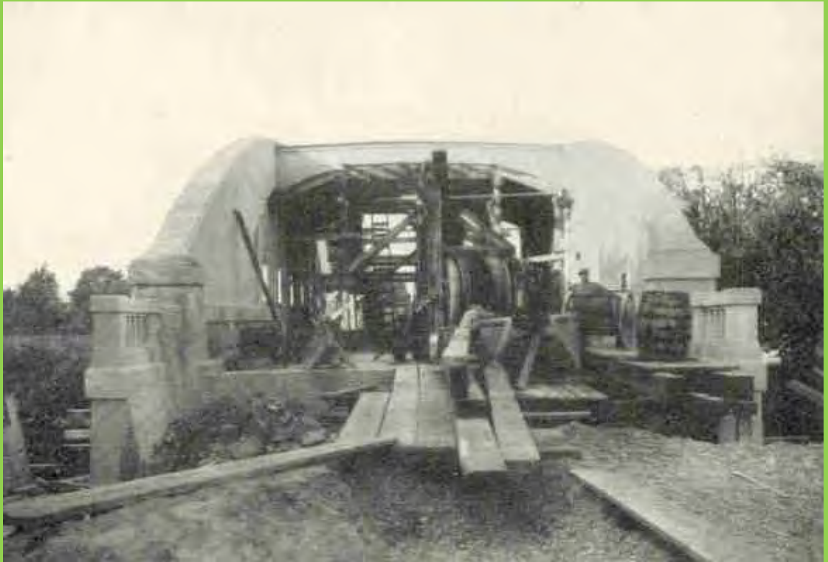
The “batch plant” on the deck with a barrel of state supplied cement
