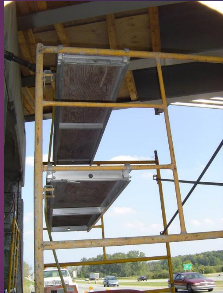
Scaffold not fully planked.
