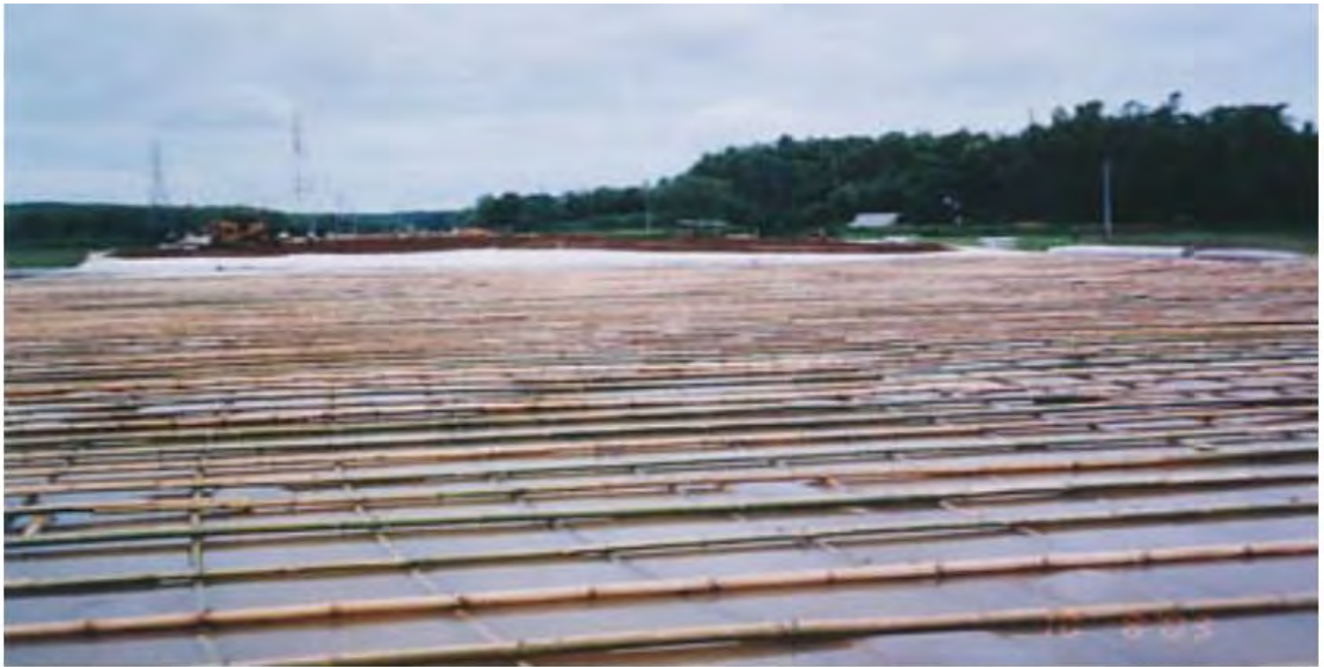
Bamboo Fascine laid over Separator Geotextile TS-80 Controlled Stage Construction of Geotextile Reinforced Embankment of 7.0 m high over a 9.0 m of extremely soft soil using high tensile strength Geotextile
