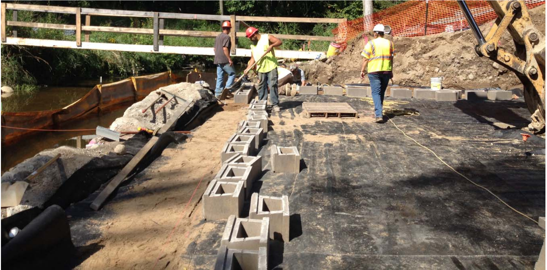
GRS ABUTMENT PROJECT PLANNING – KEEFER HIGHWAY BRIDGE PAUL SPITZLEY - IONIA COUNTY ROAD COMMISSION
