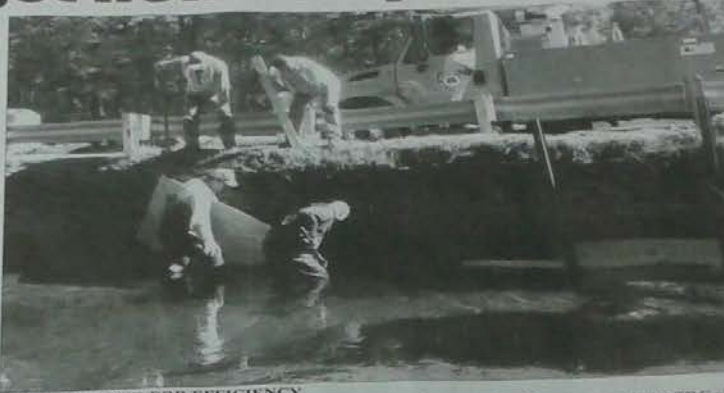
TUCK AWARDED FOR EFFICIENCY Foreman Dave Tuck was awarded the efficiency award for producing a preventative maintenance bridge/culvert program for the road commission. He said as the RCRC didn't have a plan in place he took
