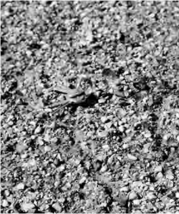
Severe raveling with ▼ extreme loss of aggregate.
