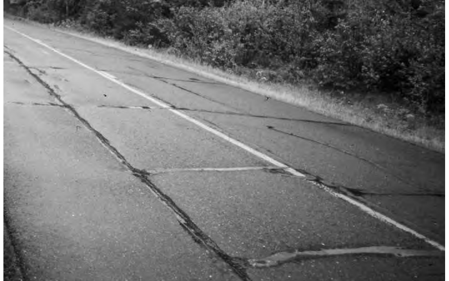
► Concrete joints reflected through bituminous overlay.
