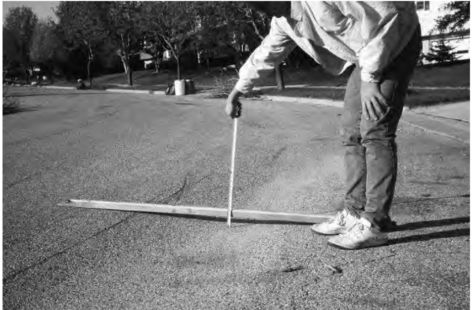
► Severe settling from utility trench.
