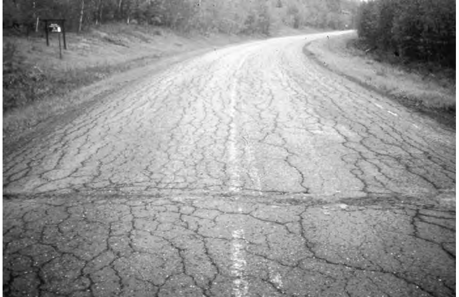
► Extensive alligator cracking. Pulverize and rebuild.
