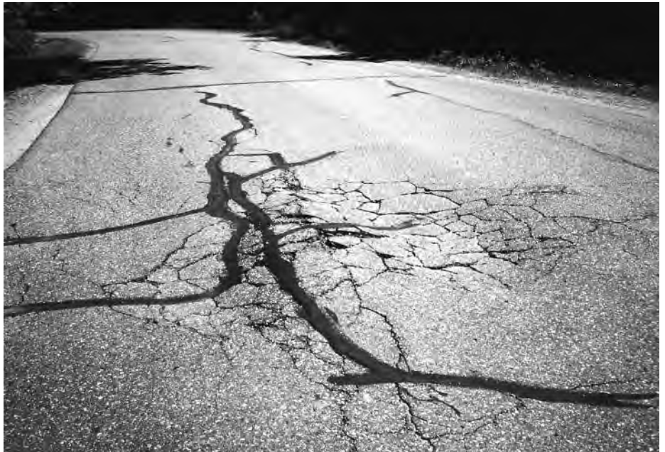
► Frost heave damage from spring break-up.
