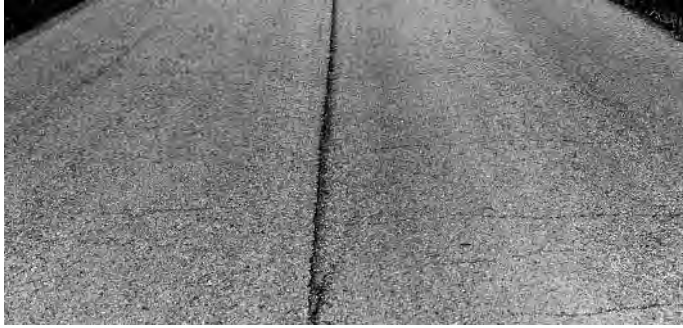
Centerline crack (still tight). ▶
