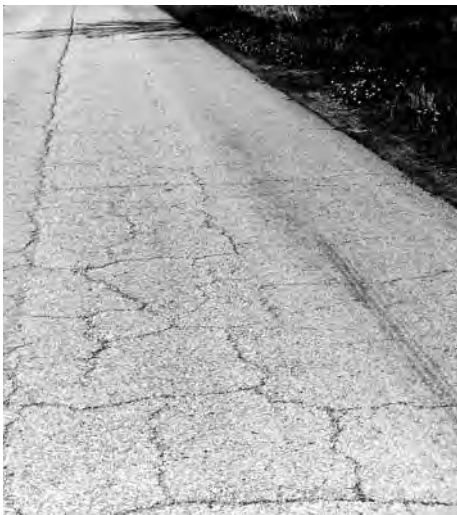
▲ Extensive block cracking in an irregular pattern.
