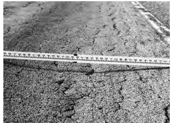
▲ Severe rutting. Strengthen base and reconstruct.
