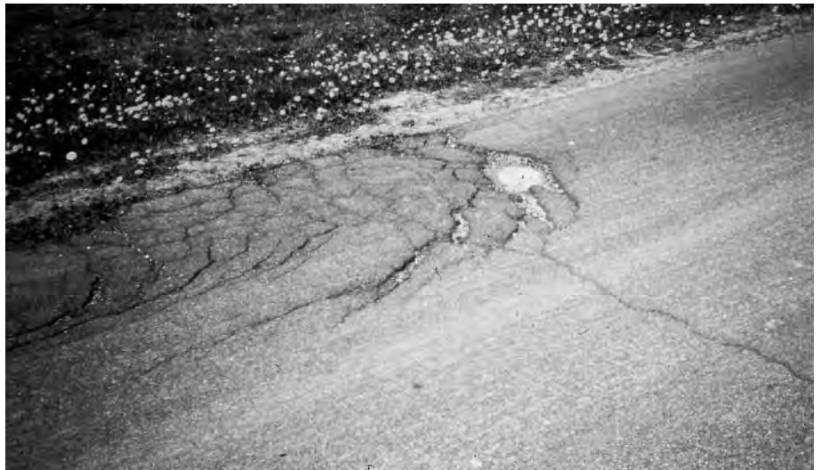
► Crescent-shaped cracks characteristic of slippage.
