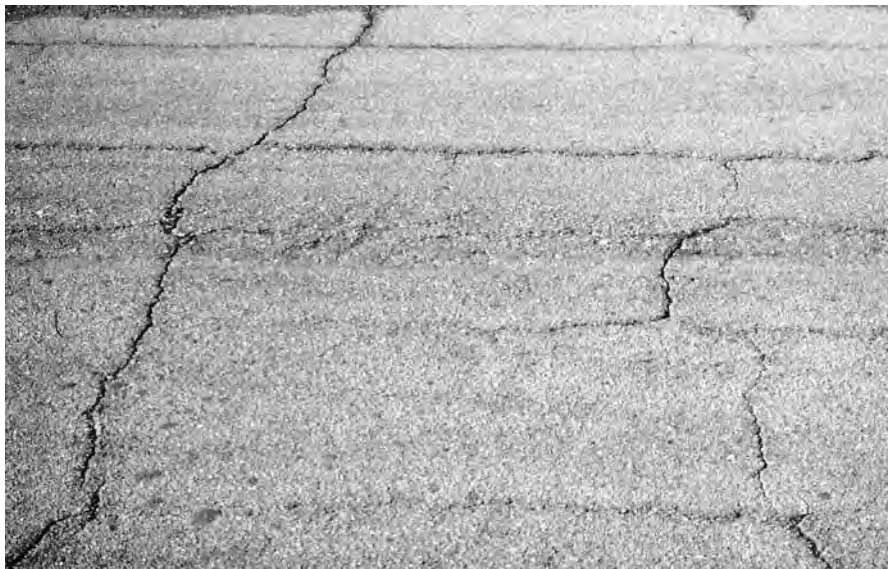
▶ Intermediate-size block cracking, 1'-5' across with open cracks.
